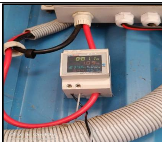
Fig. 22. Controller of solar PV system
