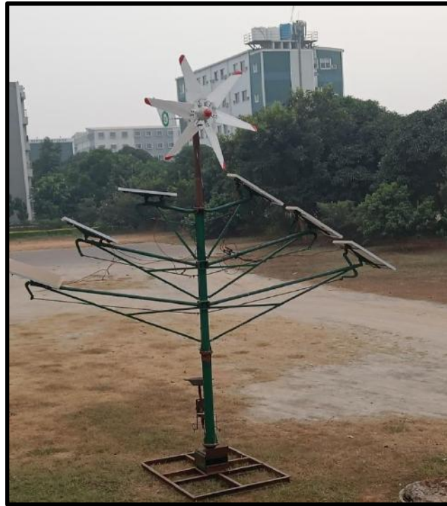
Fig. 15. Installed Microgrid inside campus
