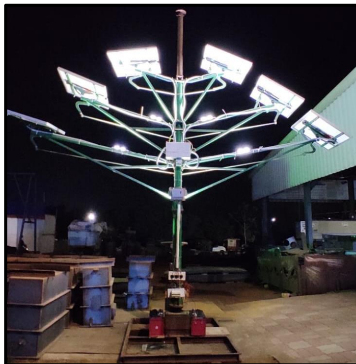
Fig. 18. Working of the installed solar tree inside campus
